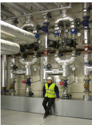
one of the realised installations
